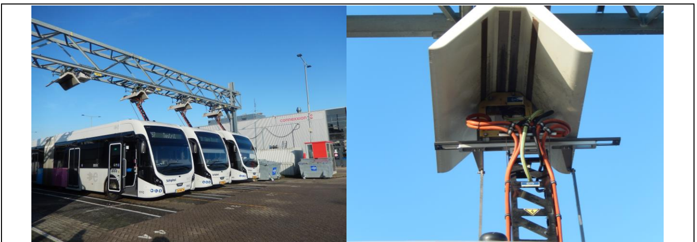
Figure 1: Battery electric buses at charging station in Schiphol Airport
