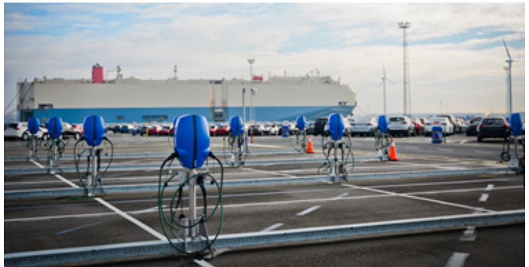
Figure 3: ICO Zeebrugge – more than 300 charging points installed (Source: ICO and CKS)
