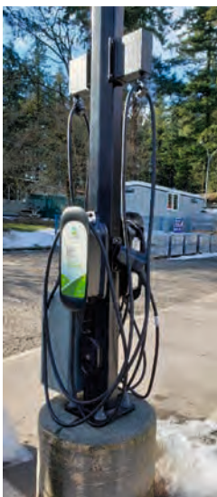
Figure 7: Streetlight mounted EV charger (Source: BCIT)
