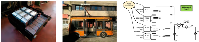
Figure 1: Storage system on board the bus (left), bus equipped with pantograph (middle) and electric schematic of the charging station (Source: ENEA)
