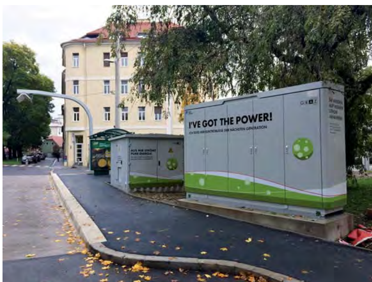
Figure 4: Fact charging integrated in bus station and grid connection in Graz (Source: Holding Graz Linien)
