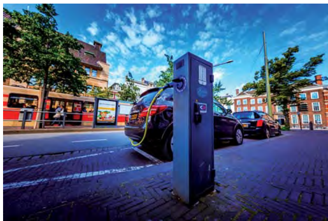
Figure 1: Charging in the Netherlands (Source: Living Lab Smart Charging, photo: Bas Stoffelsen)
