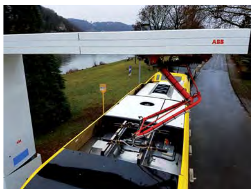
Figure 14: Opportunity charging station in Namur (Source: ABB)
