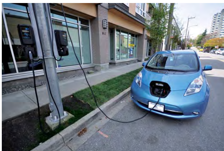
Figure 1: Streetlight integrated, curbside charging in front of a MURB in the City of New Westminster, British Columbia (Source: BCIT)
