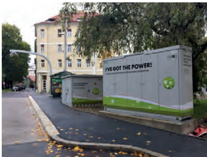
Figure 4: Fact charging integrated in bus station and grid connection in Graz (Source: Holding Graz Linien)
