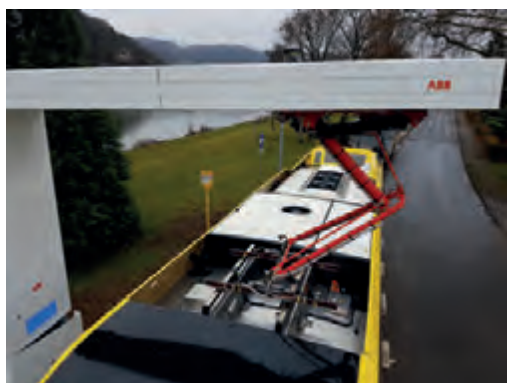
Figure 21: Opportunity charging station in Namur (Source: ABB)
