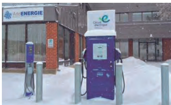
Figure 4: Level 2 and DCFC charging stations installed in front of AddÉnergie's headquarters in Québec City (Image courtesy of AddÉnergie).
