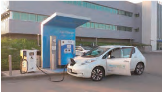
Figure 5: BC Hydro EV Charge Park at Powertech Labs – Multi-DC Fast Charger Station for Advanced Operations Testing (Image courtesy of BC Hydro).
