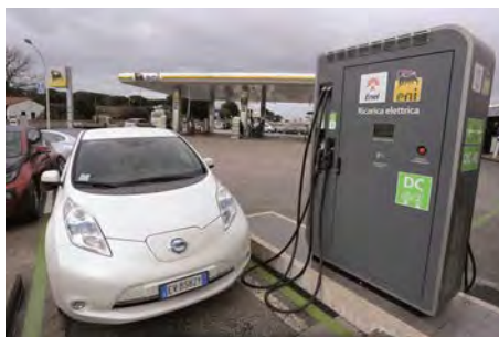
Figure 4: ENEL Multistandard Charge Station at ENI Multi Fuels Station near Rome (Image courtesy of ENEL)
