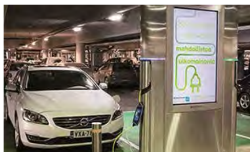
Figure 1: Charging station and digital advertising platform merged by Ensto and Symbicon
