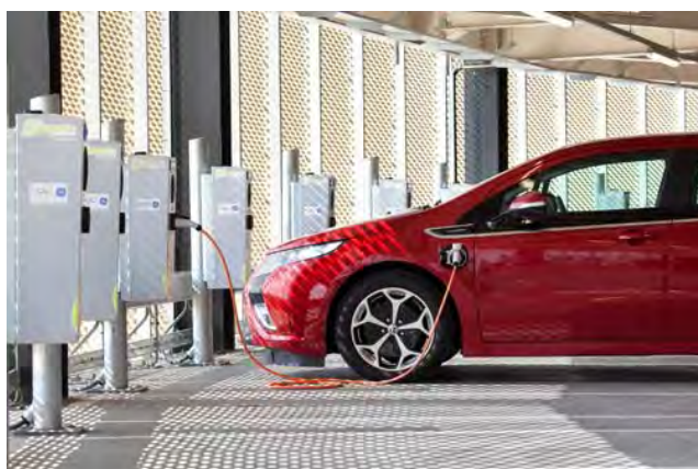
Fig. 31.2 Multi-point recharging site at Olympic Park in London.
