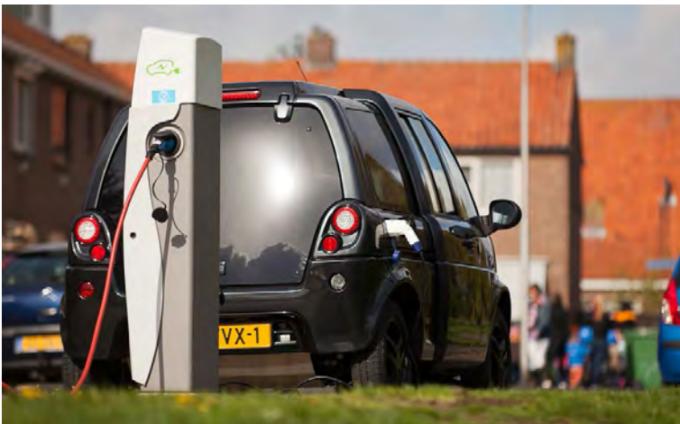
Fig. 22.1 E-laad uses an open charge point protocol (OCPP), which is an open protocol between charging stations and a central management system. The protocol started as an initiative from E-Laad foundation in the Netherlands, aiming to create an open communication standard that would allow charging stations and central systems from different vendors to easily communicate with each other.
