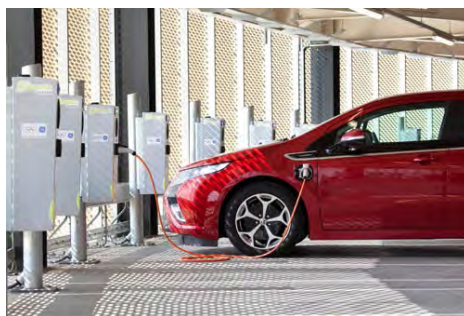
Fig. 28.2 Multi-point Recharging Site at Olympic Park in London.
