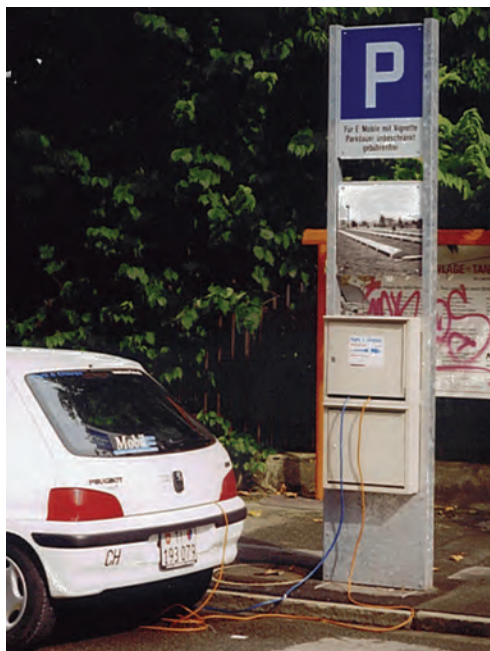
Fig. 26.3 Park & charge facility at the railway station in Thun. (Photo: Solarcenter Muntwyler.)
