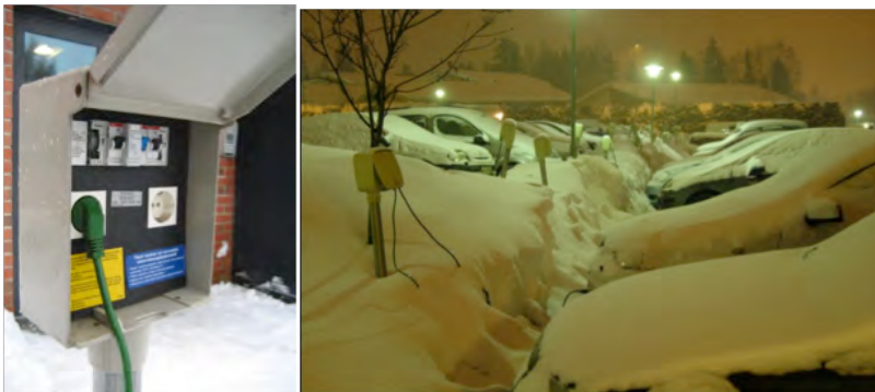
Fig. 17.2 Block heater pole (left), and view from the car parking area of a row house condominium (right). Block heater poles typically have 2-hour timers; the starting time is selected by the user, and the heating time is fixed for 2 hours from the start.
