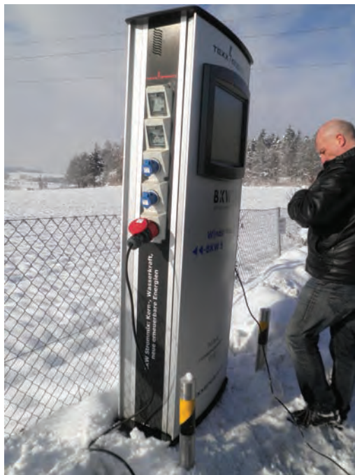
Fig. 27.10 TEXX fast-charging freeway facility service station Grauholz. (Photo: Solarcenter Muntwyler.)
