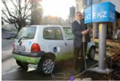
Fig. 24.9 EKZ Charging station in Zurich. (Photo supplied by EKZ.)
