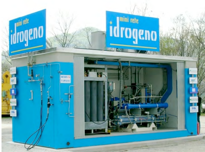
Fig. 19.4 ENEA Brasimone H 2 refuelling station for testing components. (Photo courtesy ENEA.)
